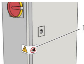
Fig. 66: Seal on switch cabinet
